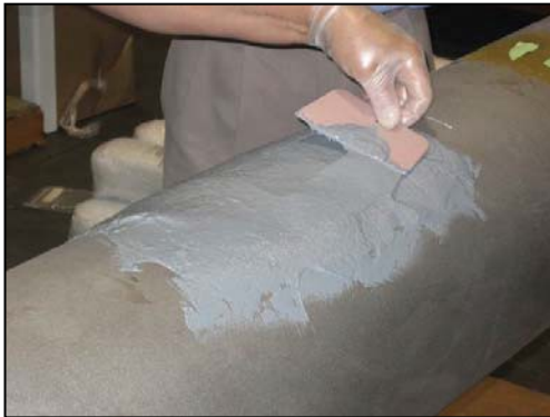
Fig. 3 – The defect must be completely filled in and the compound must be smoothed and leveled out. Remove high spots and fill any low spots
