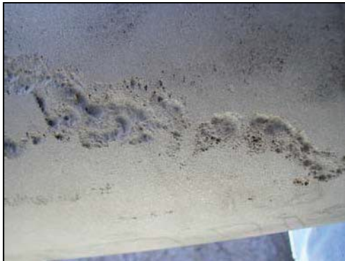
Fig. 1 – The sandblasting done on this line revealed more damage than was visible during the initial inspection. Proper cleaning is essential to a sound repair.
