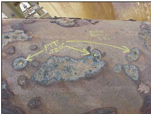
Fig. 2 – Surface preparation as shown is generally unacceptable. In cases where the pipe cannot be properly cleaned, it should be noted that the final ultimate properties of the composite layup may be compromised (such as bonding to the steel surface).
