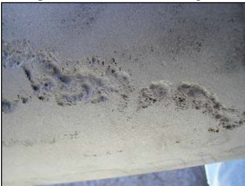
Fig. 1 – The sandblasting done on this line revealed more damage than was visible during the initial inspection. Proper cleaning is essential to a sound repair.
