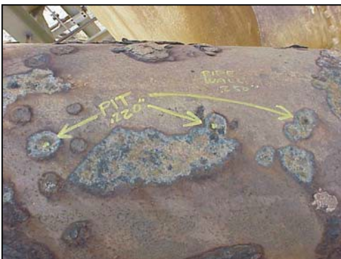
Fig. 2 – Surface preparation as shown is generally unacceptable. In cases where the pipe cannot be properly cleaned, it should be noted that the final ultimate properties of the composite layup may be compromised (such as bonding to the steel surface).
