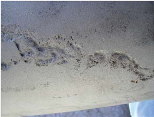
Fig. 1 – The sandblasting done on this line revealed more damage than was visible during the initial inspection. Proper cleaning is essential to a sound repair.
