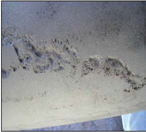
Fig. 1 – The sandblasting done on this line revealed more damage than was visible during the initial inspection. Proper cleaning is essential to a sound repair.
