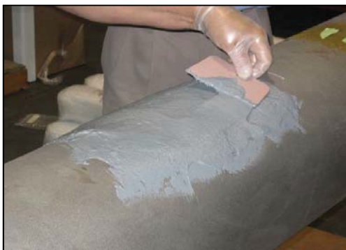
The defect must be completely filled in and the compound must be smoothed and leveled out. Remove high spots and fill any low spots.
