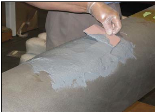
The defect must be completely filled in and the compound must be smoothed and leveled out. Remove high spots and fill any low spots.
