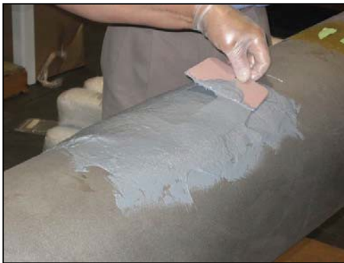
Fig. 3 – The defect must be completely filled in and the compound must be smoothed and leveled out. Remove high spots and fill any low spots
