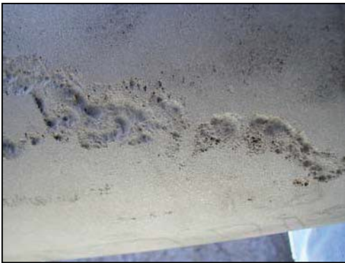
Fig. 1 – The sandblasting done on this line revealed more damage than was visible during the initial inspection. Proper cleaning is essential to a sound repair.
